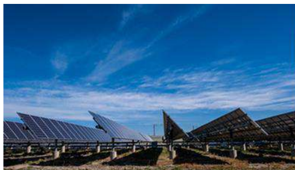
Fig.1: Solar photovoltaic system installed at Denver International Airport. Photograph provided courtesy of Denver International Airport.
